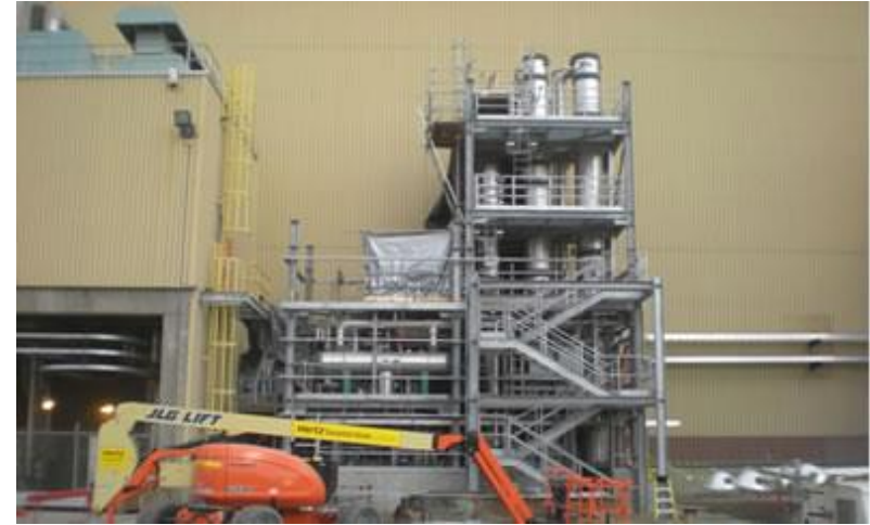
Alberta-Pacific Forest Industries Inc. , Methanol purification project, Boyle, Alberta
